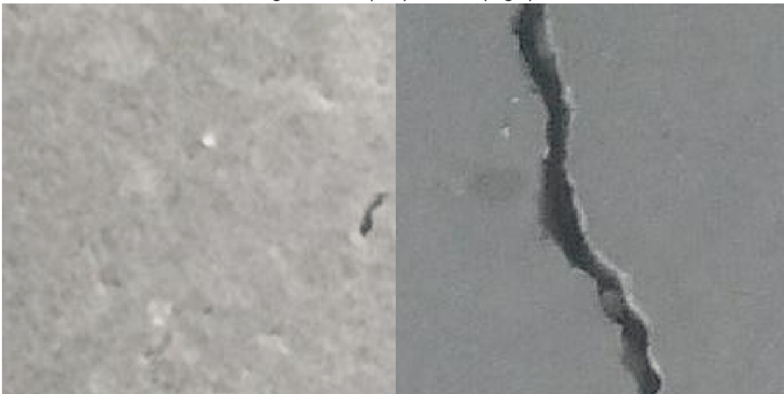
Road Images Without (Left) and with (Right) Cracks
